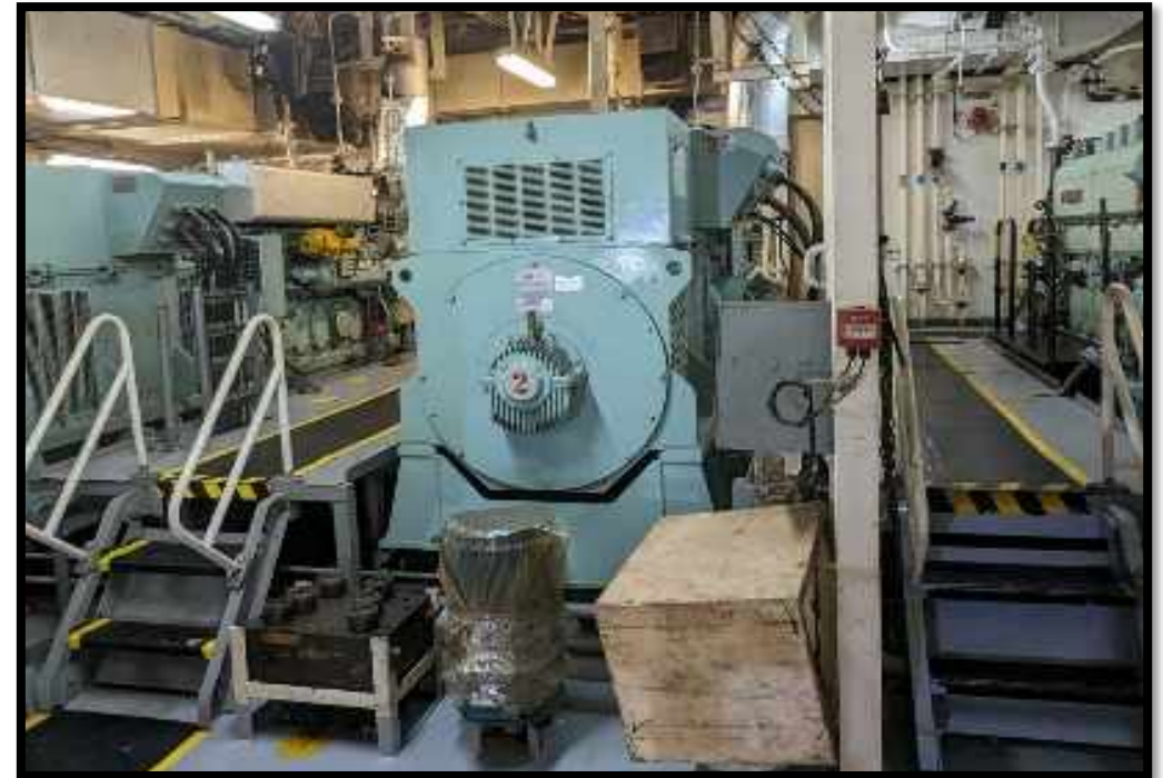
Generators (Auxiliary load)
